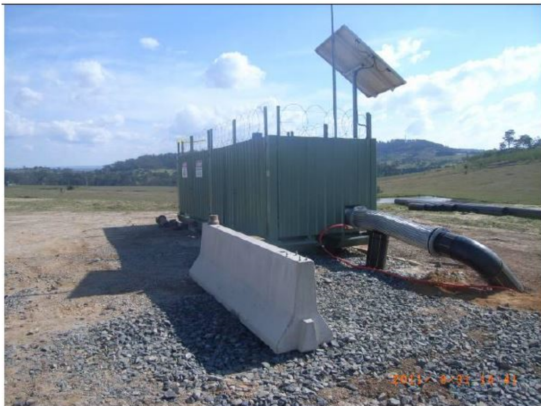
Figure 25 : Gas Extraction Plant Connected to MRD Drainage Well (Cardno, 2011)
